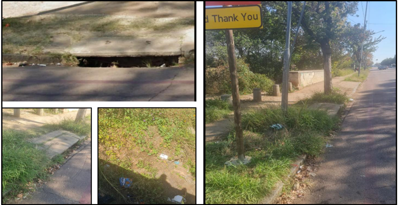
Figure 2: Photographic records of the outlet vicinity near MH01A prior to full exposure, indicating the available working corridor, existing cover slabs/structures, and proximity to the vegetated embankment and receiving environment.
